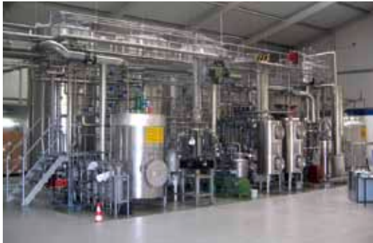
Biodiesel Renewable energy Cogeneration unit plants
