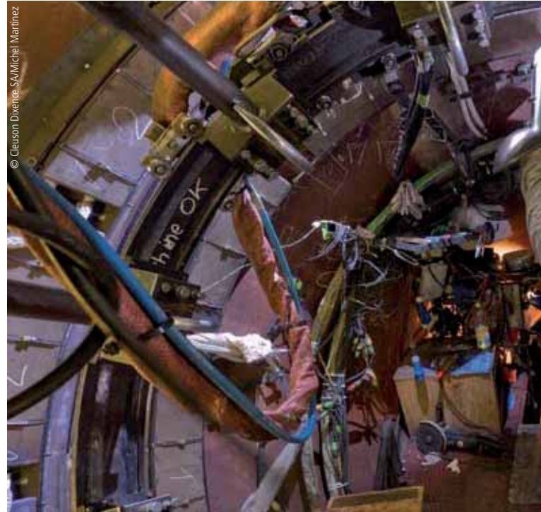
A prestigious project completed by MCE AG: the replacement of the pressure shaft cladding at the Cleuson-Dixence hydropower station in the Swiss canton of Wallis.
