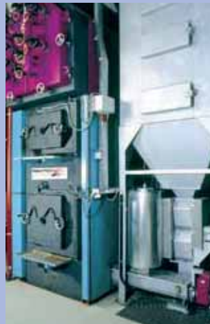
600 kW hydraulic grate firing plant from POLYTECHNIK.
